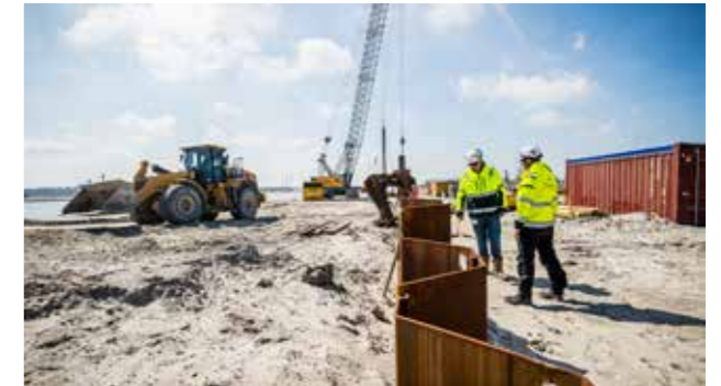
Before excavation, sheet piles were placed around the future German tunnel portal
