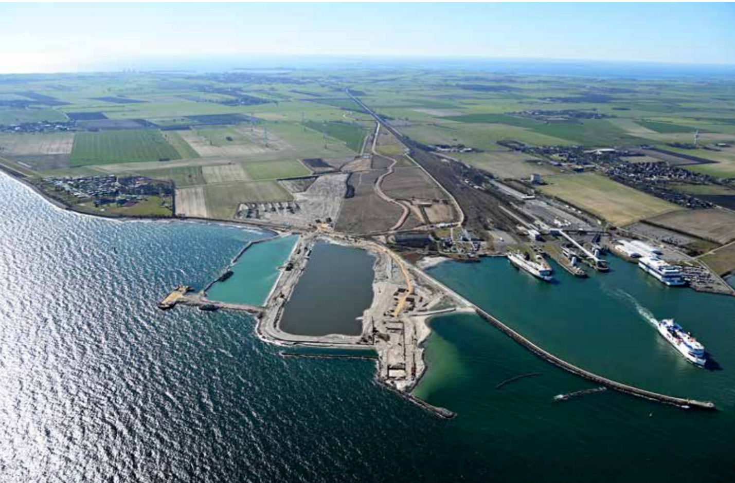
The German construction site near Puttgarden on the island of Fehmarn: work is currently underway on the German portal and the working harbour
