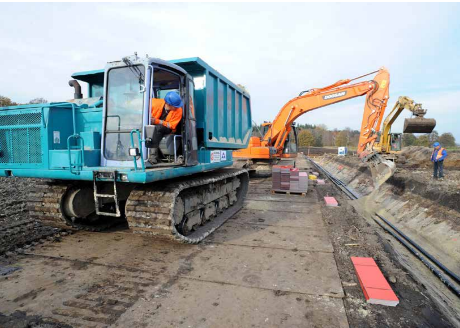
Cable laying for a high-voltage transmission line: The special cables laid in the excavated trench are first covered with a special fill before excavators refill the trench with soil
